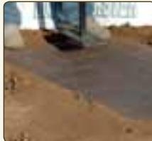
Install MoundMaster Blocks, moisten, tamp, then fully water and allow to soak in for 20 minutes.
